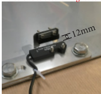
Figure 14 - Magnetic burst sensor proper installation
